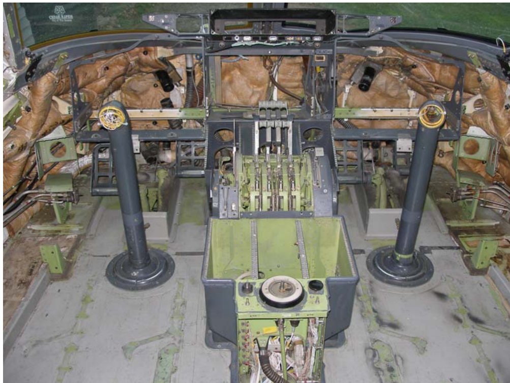
With glareshield and all wiring removed, access to the aeroduct tubing Could be gained and replaced and deep cleaning could finally begin
