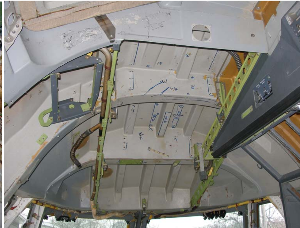
The removal of all the overhead wiring can be seen here now that the pilot's overhead panel and circuit breaker panels are removed.
