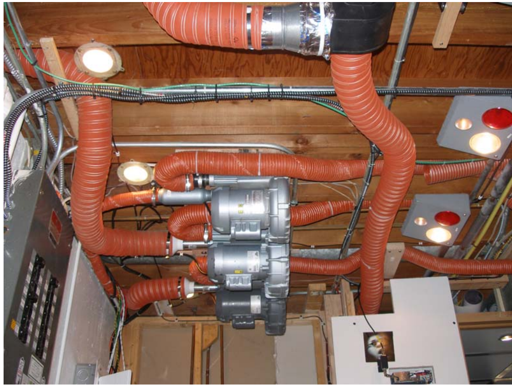
Three regenerative high capacity blowers were mounted to the Ceiling and drew air from the house's air conditioning ductwork out to The flight deck's original complex ductwork and plenum system inputs
